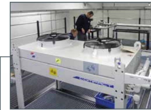
Dry cooling tower
