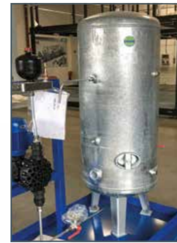
Part of the thermal reactor
